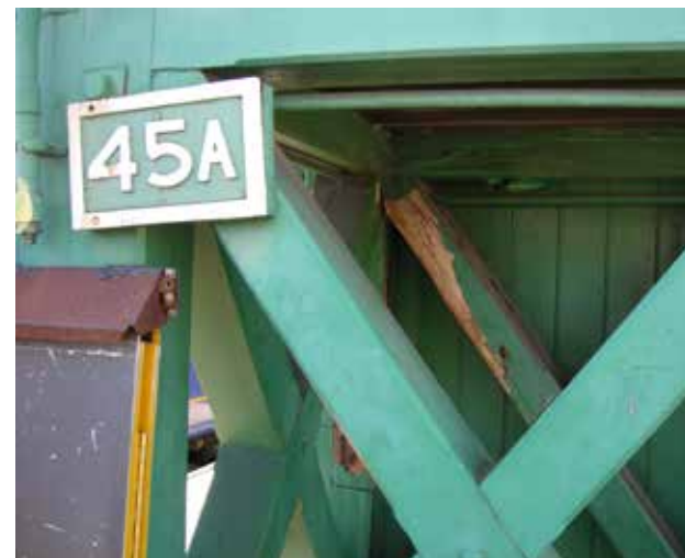
Rot visible in trestle legs on platform 1
